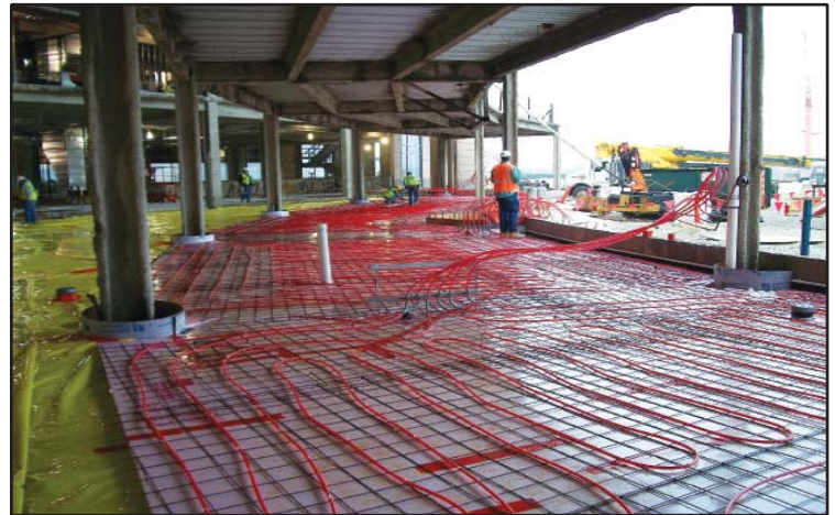
Above: Pex tubing for in-floor radiant heat at the Silver Cross Hospital Entry.
